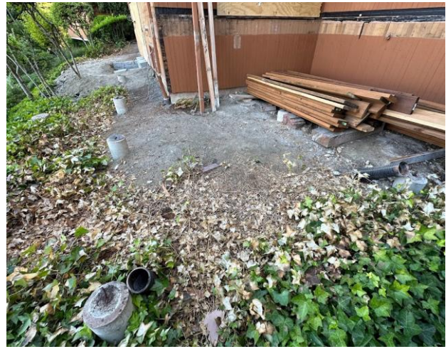
Plate 2. View of the exposed soils over the replacement deck area, existing footings left in place.
