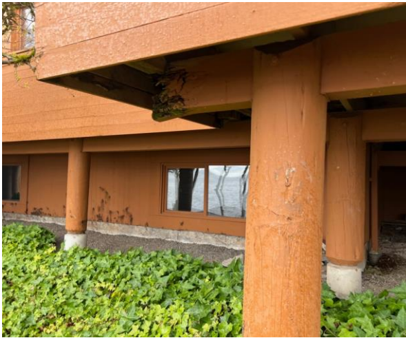
Plate 1. View of the previous deck with rotted beams and posts. Deck has since been demolished.
